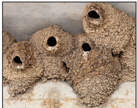
Mud nest colonies can alter the balance of structures, including pole signs, bridges, canopies, water towers, etc.
